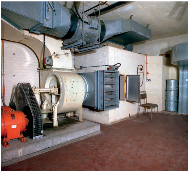
Ventilation and filter chamber in the plant room in the original war room. Three or four hundred people need a lot of air, and a clean supply without radioactive fallout contamination was vital. Filtering and pumping it would require a lot of fuel for power. Photo Nick Catford
